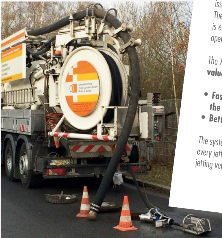
This photo was taken during a cleaning operation in a DN 600 pipe.
